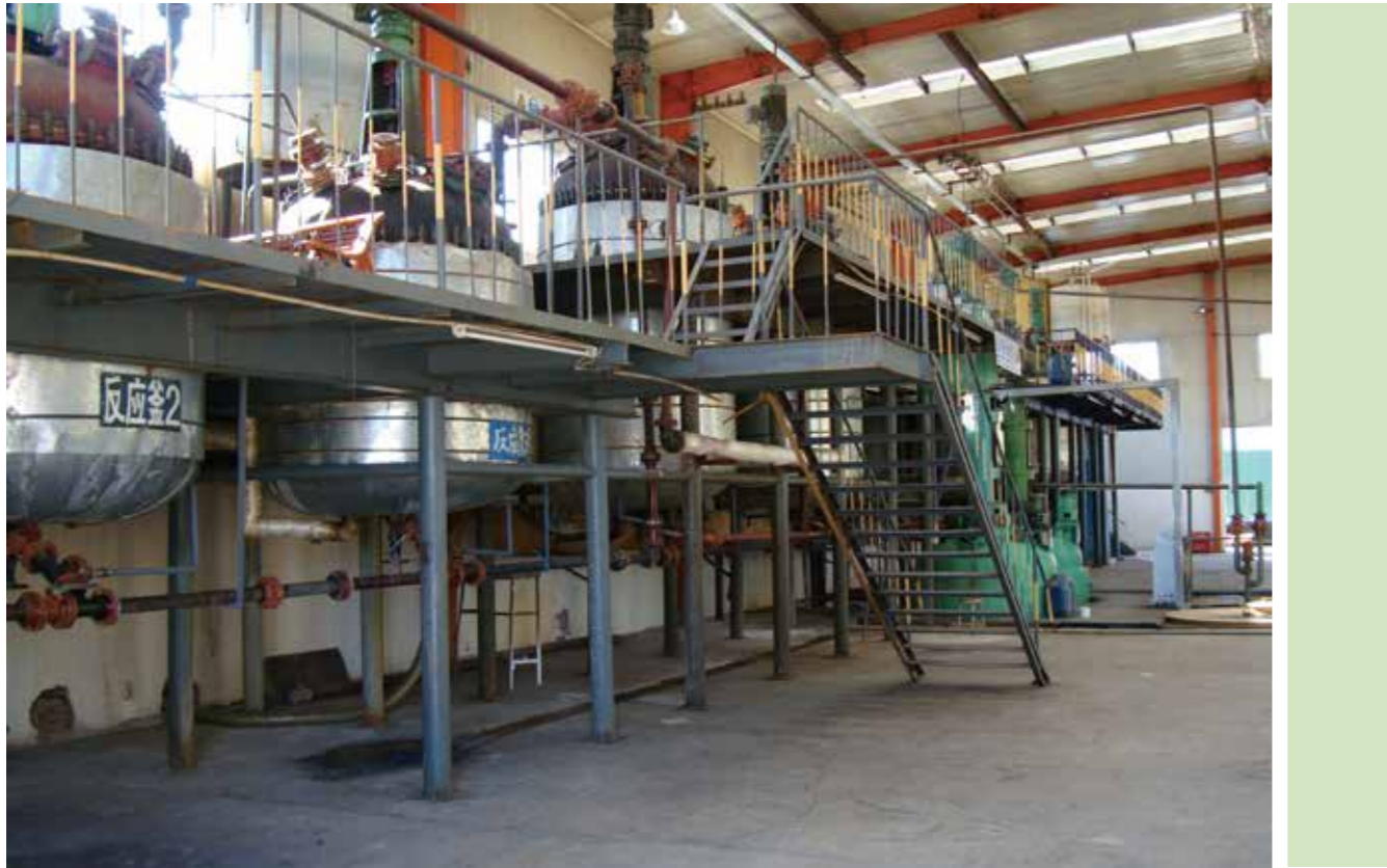
Automated Naphthalene Sulfonate Formaldehyde(SNF/NSF/PNS) of Production Line
